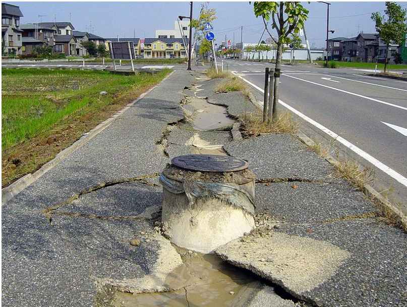
Seismic forces can lead to ground ruptures and/or subsidence. (Photo by: Tubbi)
