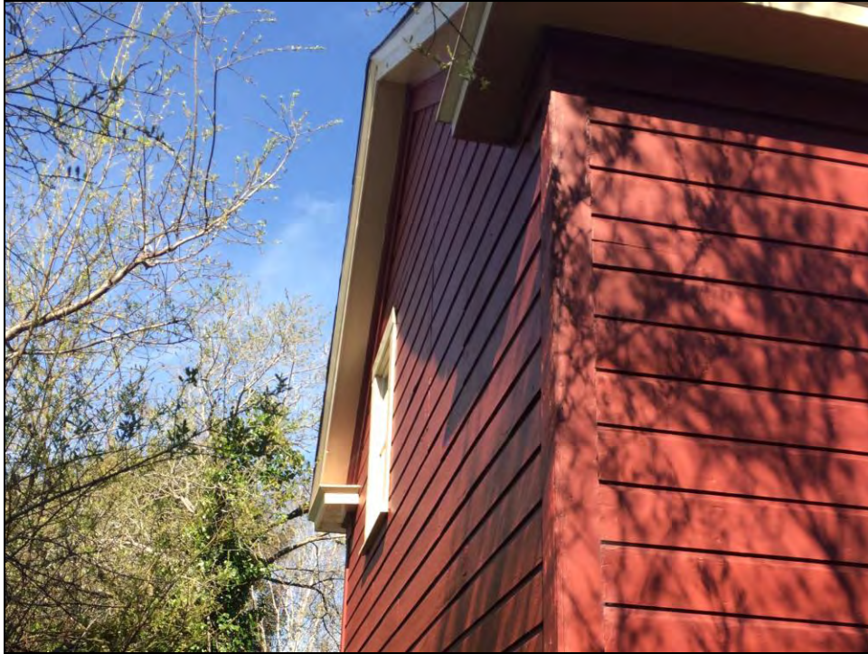
Photo 9: View across west-facing wall of Blume Bunk House, including patched former window location.
